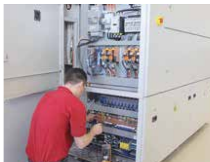
Freely accessible switching cabinet
