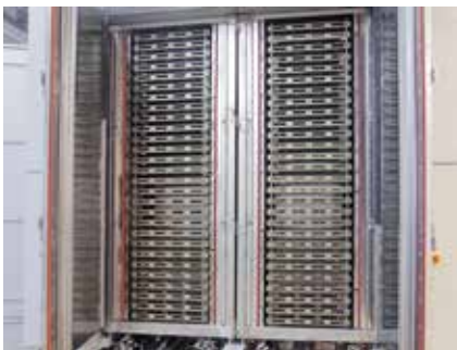
Vertical stacking principle in the process towers for receiving the goods carriers
